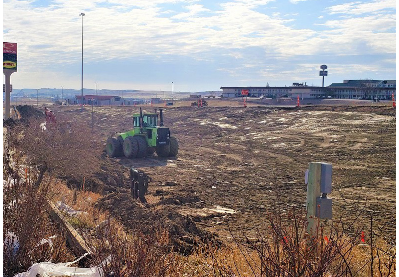
Fill is being imported at the Interstate 90 LaCrosse Street (Exit 59) westbound off ramp to widen the ramp approach to ultimately connect with the interchange over the LaCrosse Street bridge.
