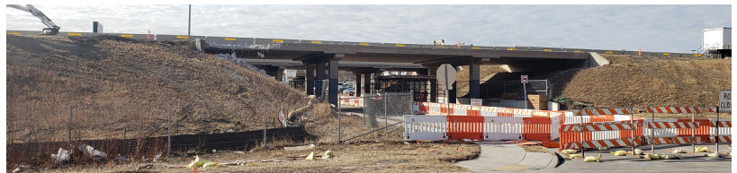
Demolition of parts of the Maple Avenue bridges is required to widen the bridge decks to accommodate one auxiliary lane in each direction. This photo also shows the temporary pedestrian route created beneath the bridges, allowing pedestrians and bicyclists safe access to and from the Rushmore Mall area.
